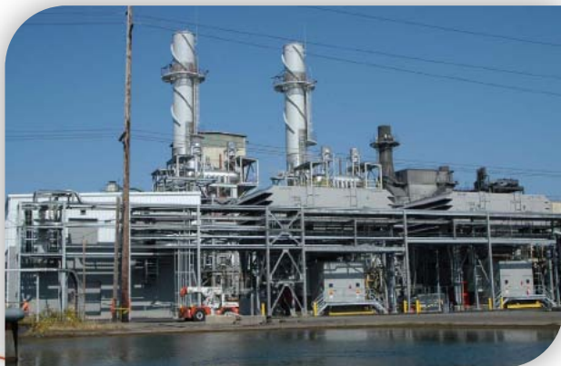
92 MW Newberg, Oregon SP Newsprint Gas Turbine CHP Plant
